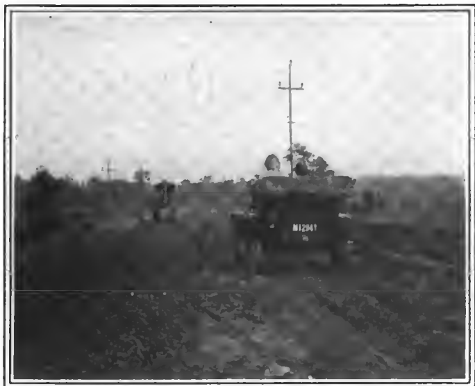
Widening new road near Blacksburg. Note the road roller and broken stone
